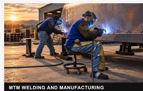
MTM WELDING AND MANUFACTURING
